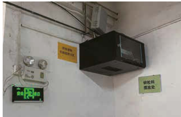
Online monitoring system for solid wastes 固體廢物線上監控系統
